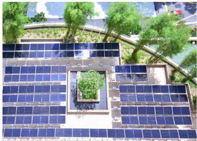
■ Solar panels installed on the roof of Ren Ci Community Hospital
